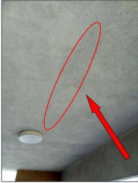
Formations of Cracks along the Joints in the roofing panel
