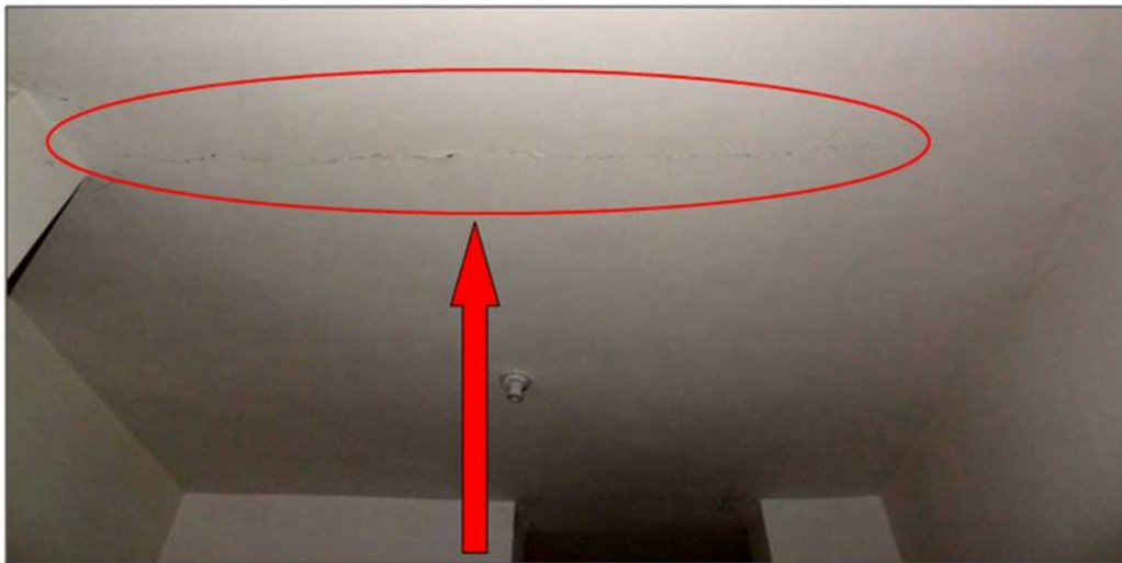
Formations of Cracks along the Joints in the roofing panel
